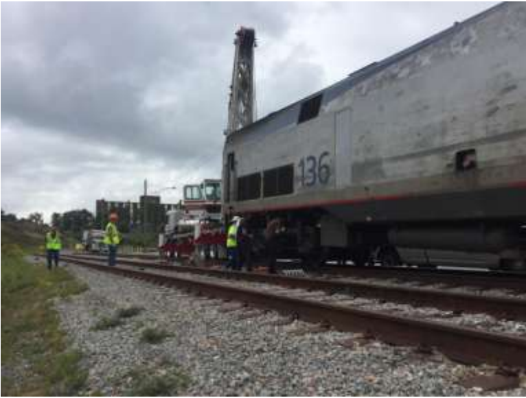
Sep. 22 - Amtrak engine 136 needed a little attention to repair a broken suspension spring. Cranemasters was called in to do the lifting of the unit on site in Lynchburg. (Rick-II Johnson)
